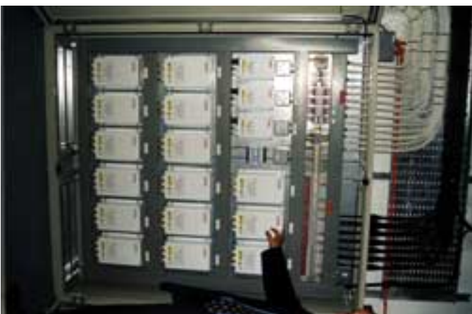
Controls at Hermiston Quays Block A twinned with Block D
