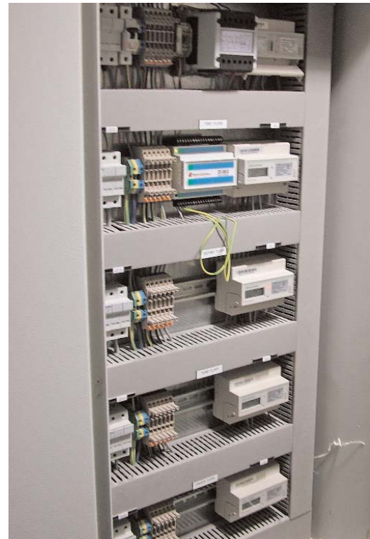
The electrical control box with the energy monitors
