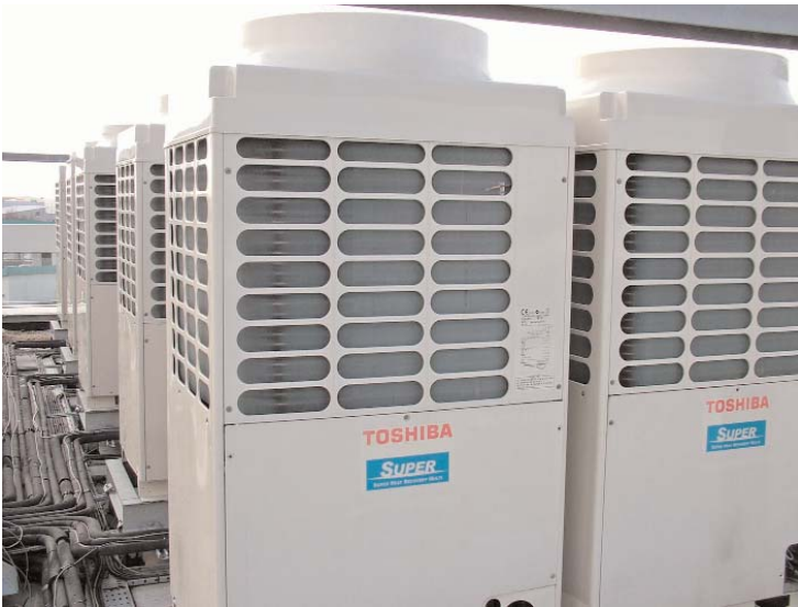
The Toshiba SHRM units on the roof
