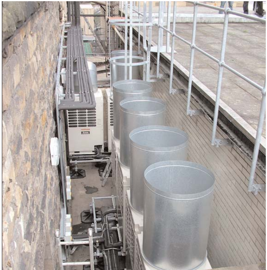
The outdoor units are discreetly sited – the cowls have proved an excellent solution
