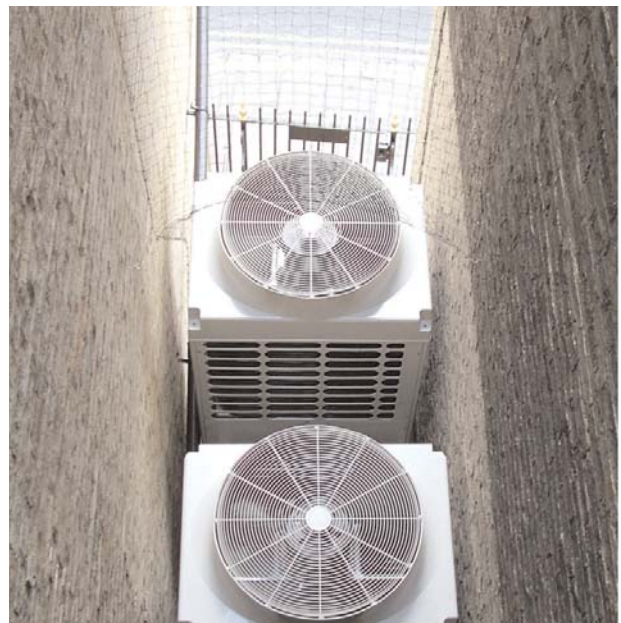
The siting of the outdoor units was approved by the local Planning Department
