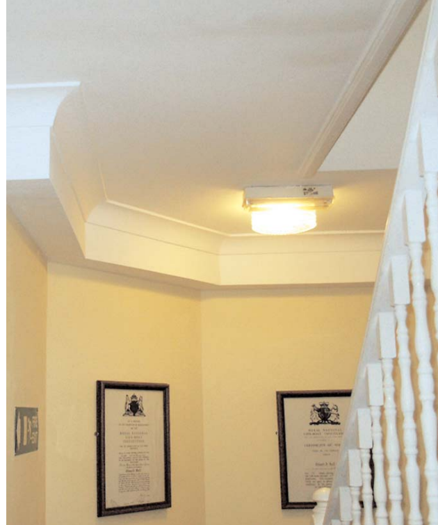
The plasterwork had to comply with the building's listed status and fire regulations
