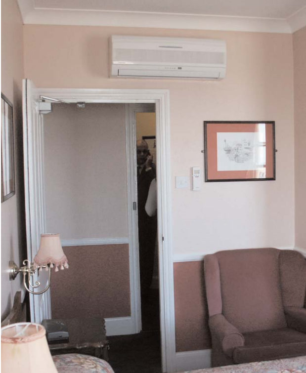
Adding air conditioning is part of a project to upgrade the suites
