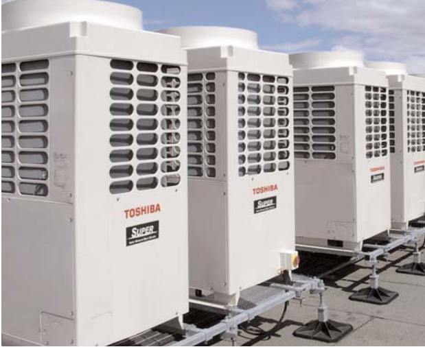
Toshiba VRF units on the roof
