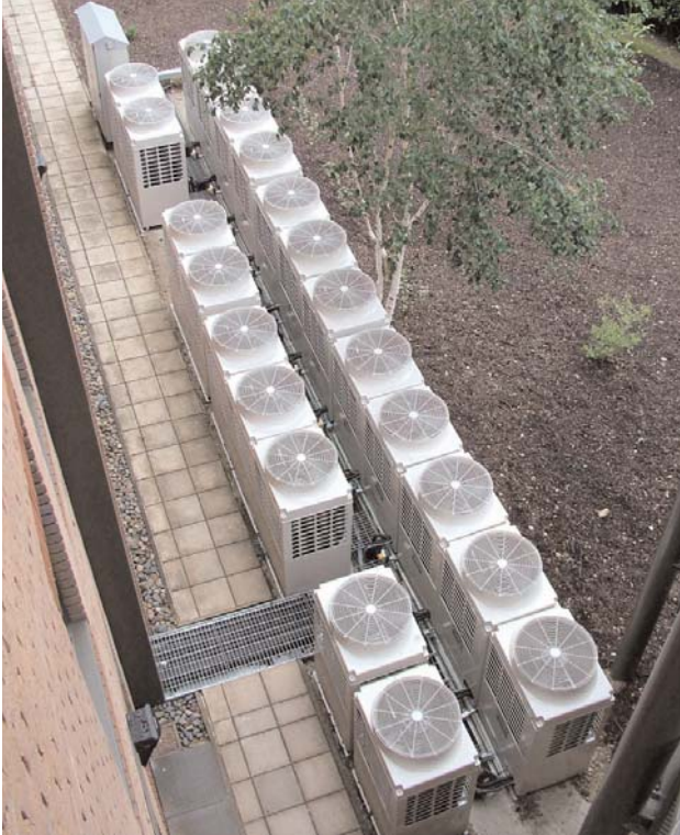
The condenser farm fits the same footprint as the previous equipment
