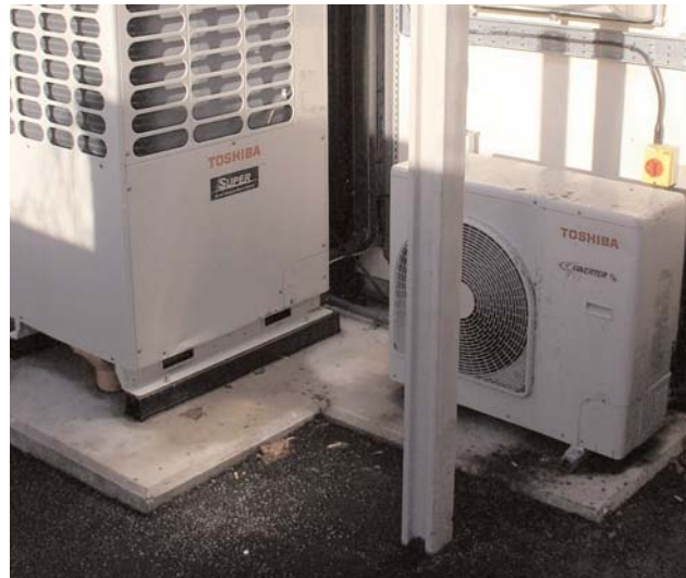
The outdoor units don't disturb the neighbours
