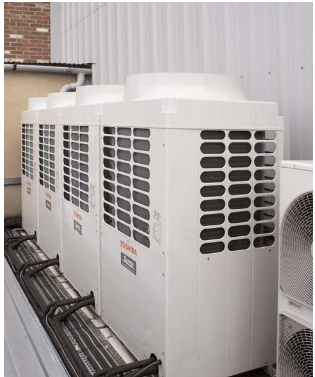
The outdoor units sited in the yard are too quiet for neighbours to notice them
