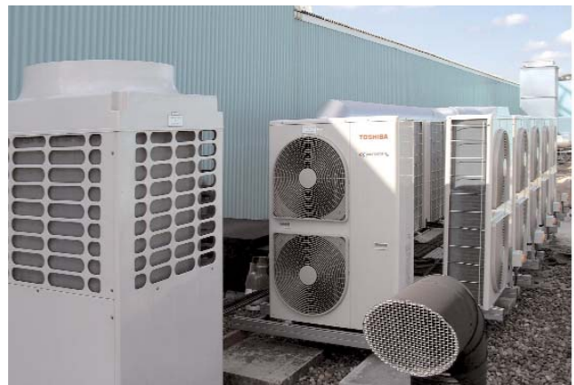
The VRF system provides flexibility for further extension of the shop unit
