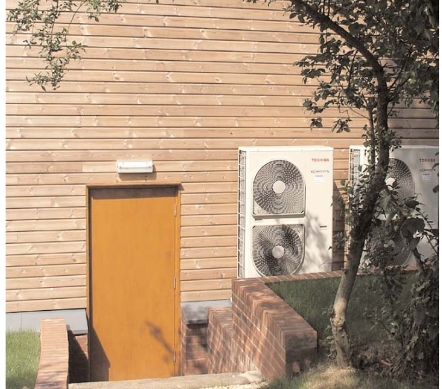
The outdoor units are discreet
