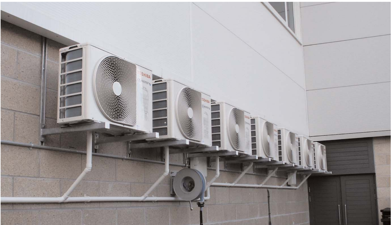
The outdoor elements are sited in a plant area
